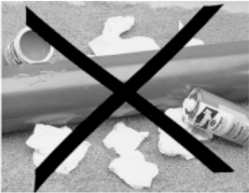
The pipe trench is not a rubbish tip
